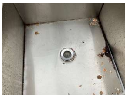
All six main washbasins were installed with sink strainers
