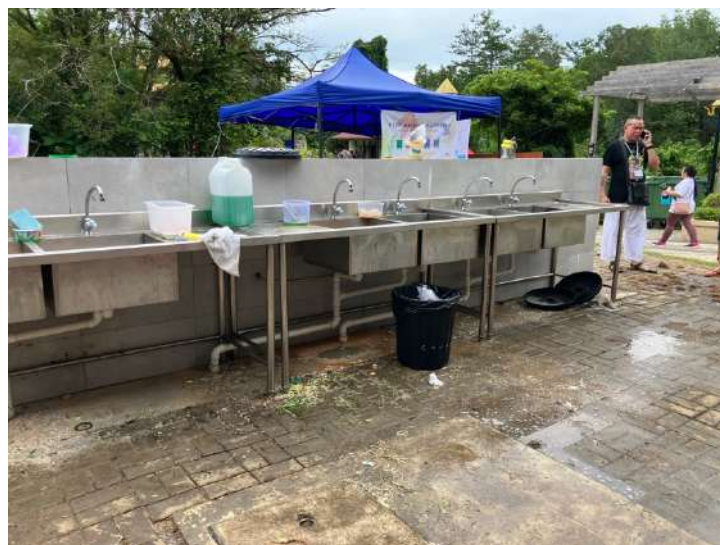
Photo 20: Contamination due to lack of proper drainage system. We plan to install more food barrels next to washbasins in the future.
