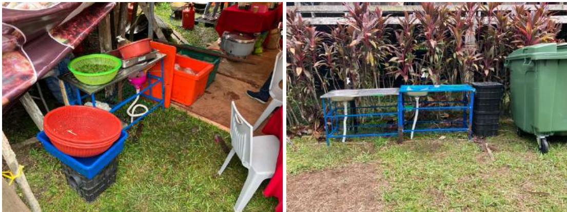
Photo 18 & 19: Three grease traps were uninstalled so we had to source out our materials for installation in the last hour before further contamination can happen.
