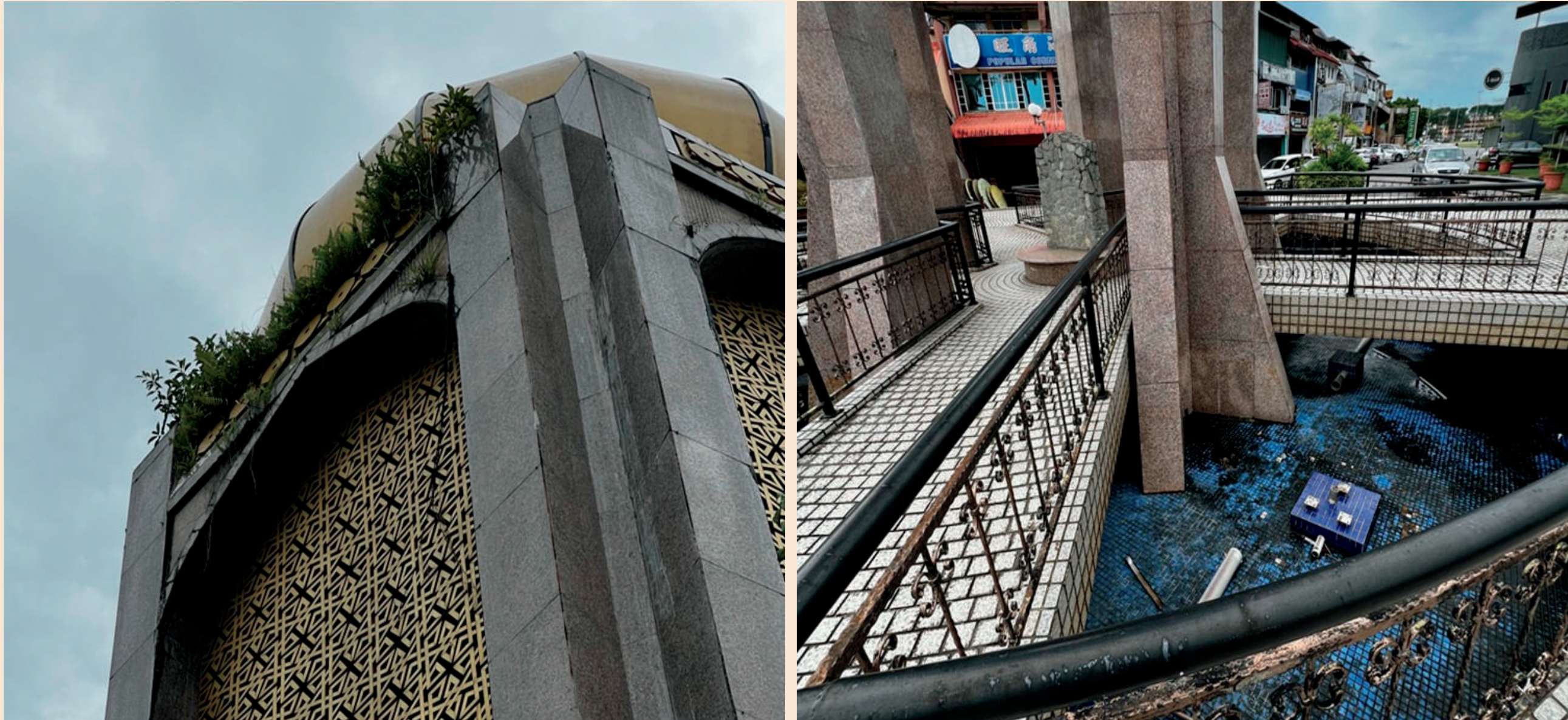
Stone Memorial Monument – No Maintenance, Water fountain not functioning, propose to add on lights to make it more attractive
